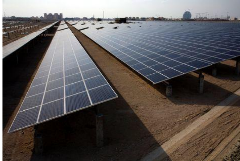
Figure (i) Nour1 100 MW solar power plant
